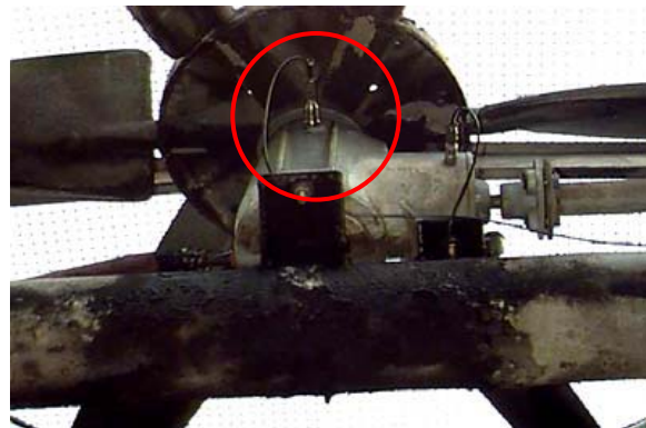
View of a large-cell fan from below, showing the mounting of a 799LF low-frequency accelerometer on the side of the gearbox.
