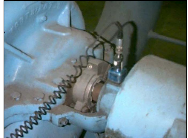
793 sensor on inboard motor bearing
