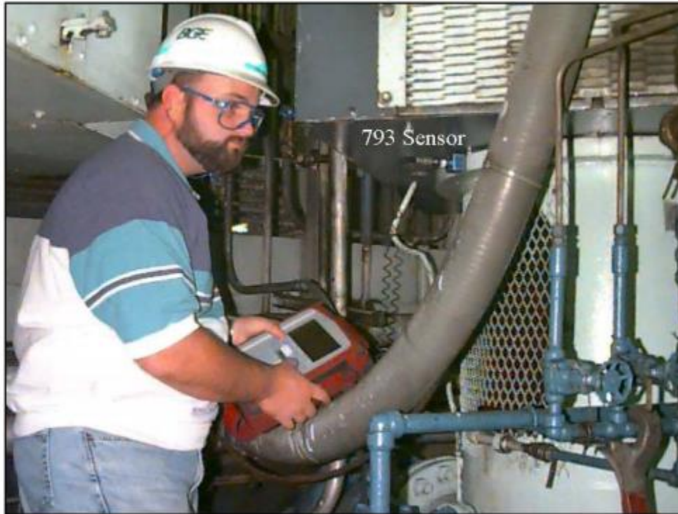
Robby Herman, plant technician, obtaining data on motor bearing
