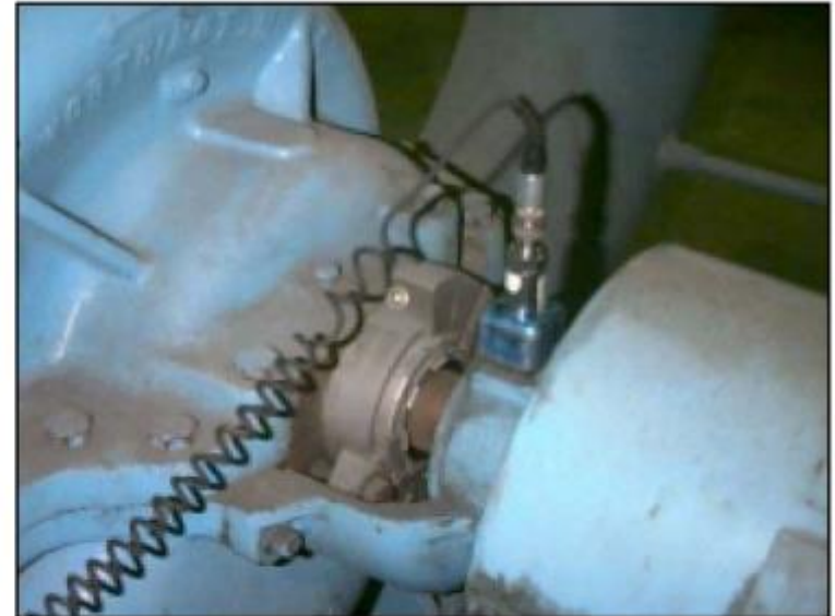
793 sensor on inboard motor bearing
